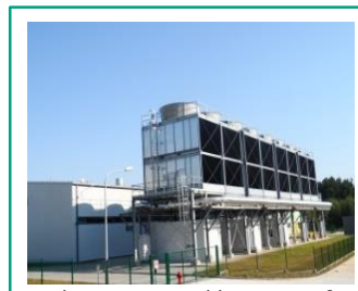
Cooling tower and heat transfer building
